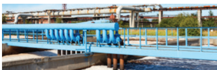
Waste Water Treatment Plant
